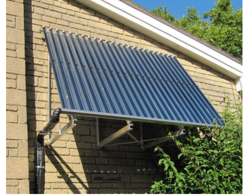
South-facing solar panel at Cranham
